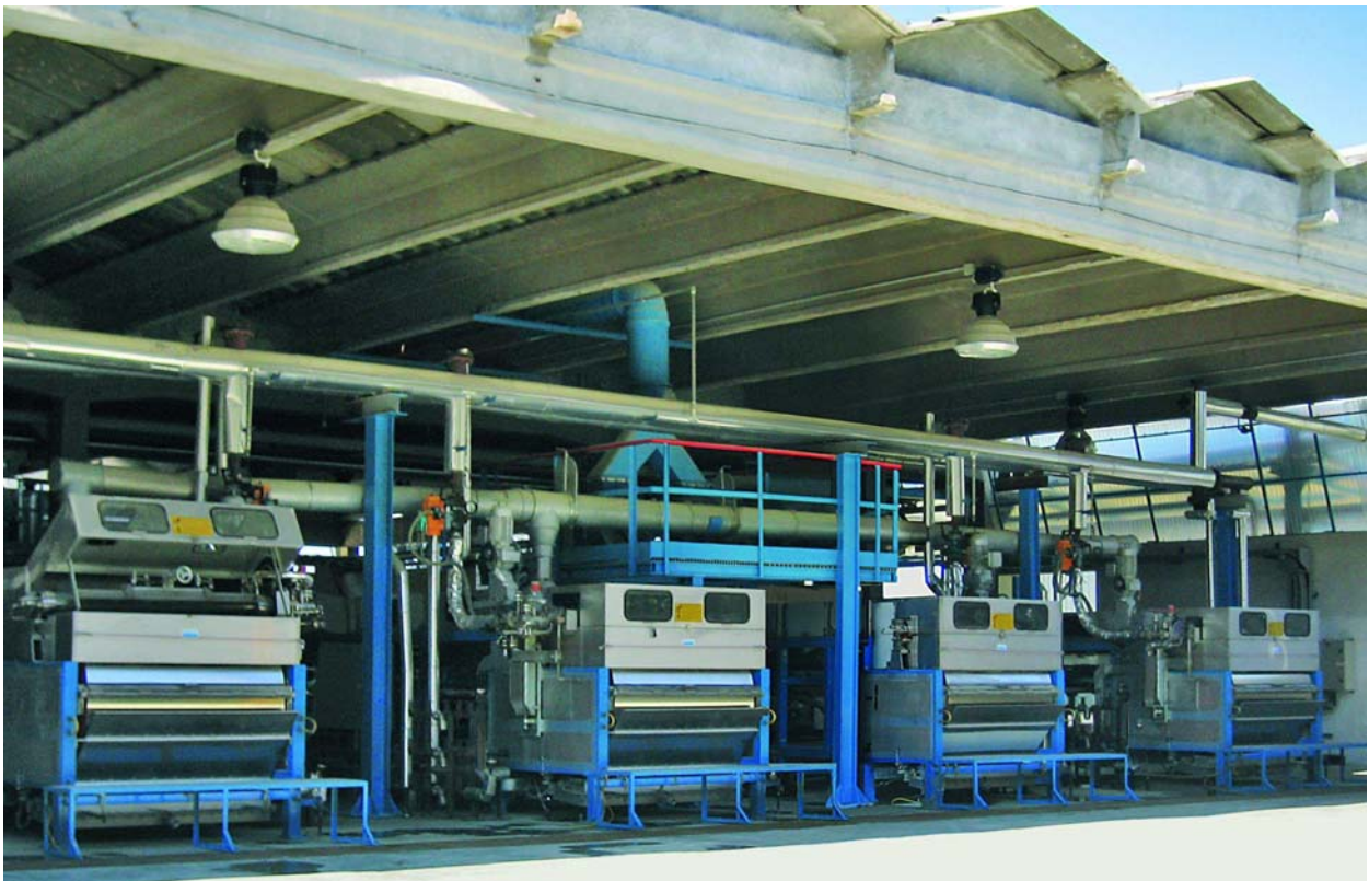
Picture 4: Front view of installation of urea plant with 4 Rotoform Units.
